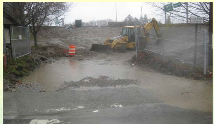
A non-compliant RIDOT construction site
