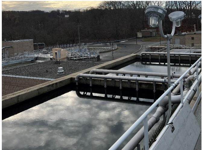
Biological aerated filters treat wastewater in West Warwick.
