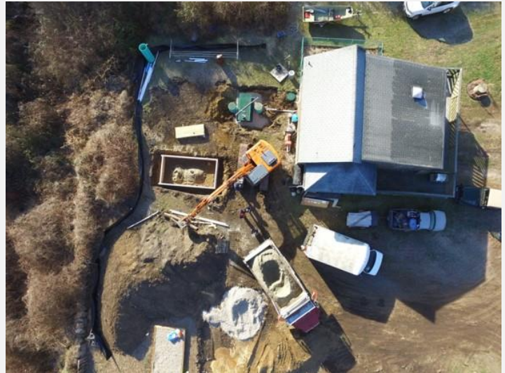
A nitrogen-reducing onsite wastewater treatment system is installed to replace a traditional septic system less than 100 yards from a coastal wetland
