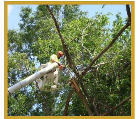
Figure 2: Arborist cleaning storm damage
